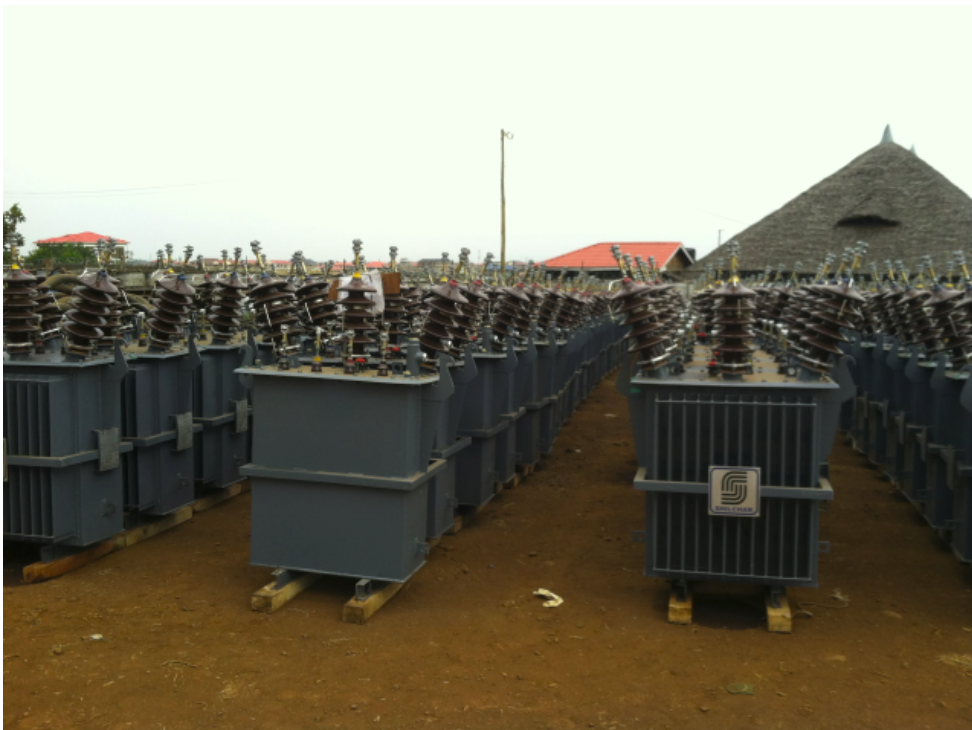
New transformers awaiting installation
